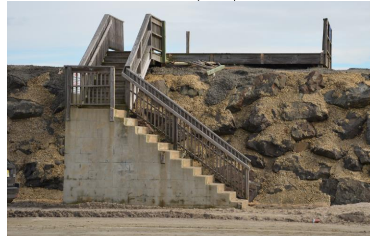
Figure 17: Damage to the Public Access Stairs at Central Avenue (1 of 3)
