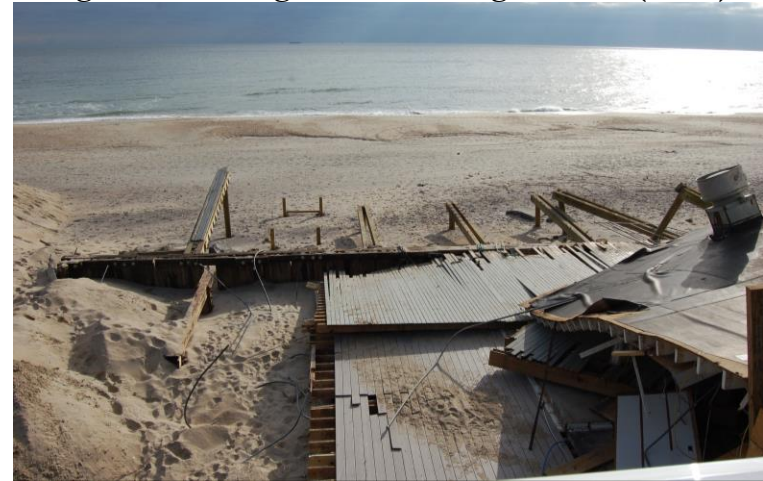
Figure 25: Damage to the Bathing Pavilion (2 of 8)
